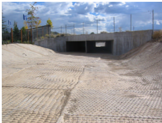
Grout-filled Fabric Revetment on Channel C
